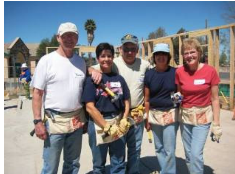
A group of volunteers prepare to help raise the walls on Habitat Tucson's first home in Marana.
